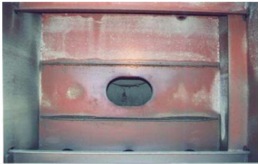
paint application, ballast tank condition after 13 years (a bulk carrier double tank is shown in this example)
