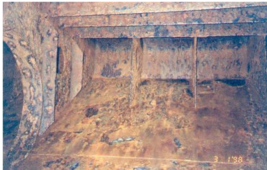
paint application, ballast tank condition after 13 years (a bulk carrier top side tank is shown in this example)
